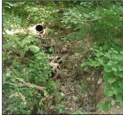
Example of erosion caused by sewers. Dumping & filling of the bluff has altered natural drainage, soil stability due to the fill materials (note rebar & concrete in photo), and the inability for vegetation to grow in given condition.
