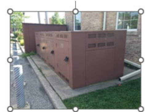
Fire Station Lighting Controller
