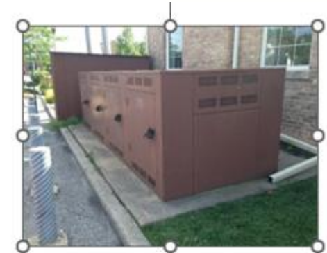
Fire Station Lighting Controller
