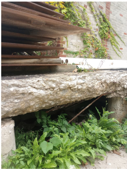
Figure 30 Exterior Platform Slab Deterioration-9
