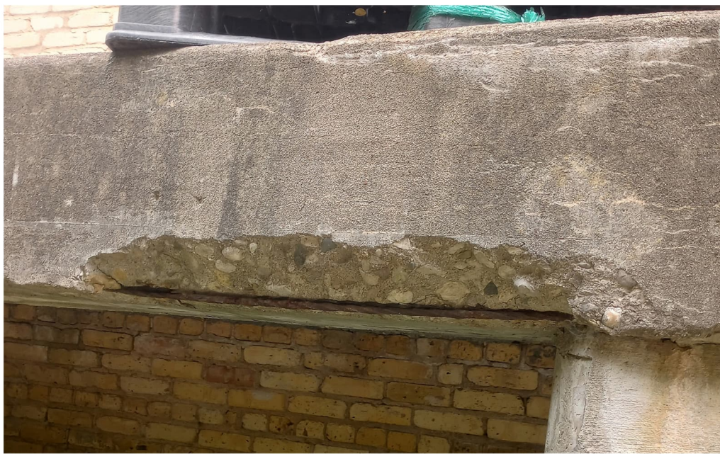
Figure 26 Exterior Platform Slab Deterioration-5
