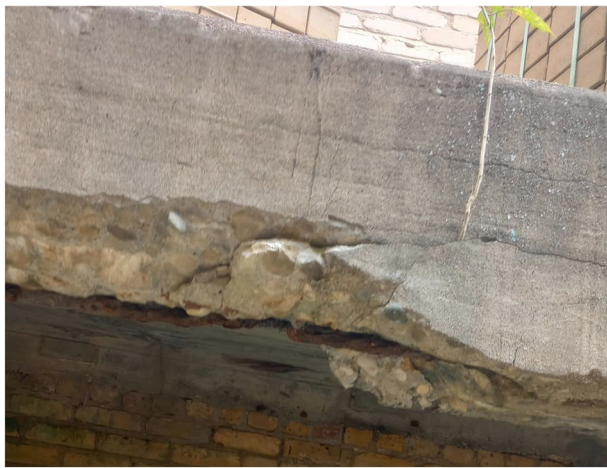
Figure 24 Exterior Platform Slab Deterioration-3
