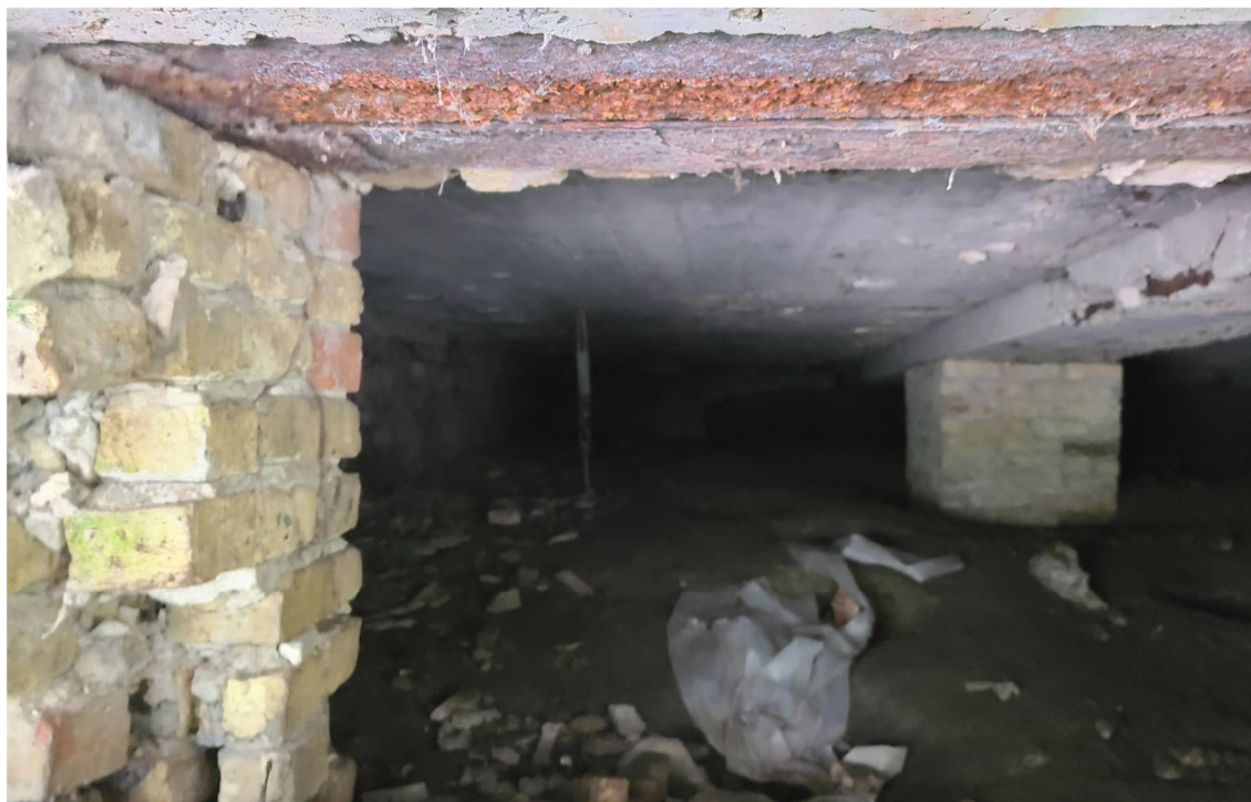
Figure 33 Corroded Steel Beam Lintel Above Access Opening
