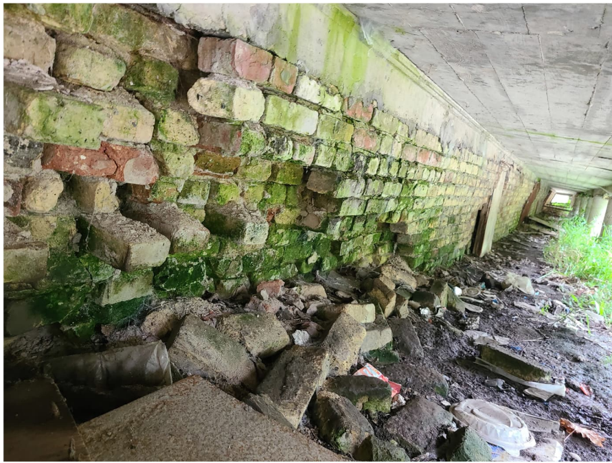
Figure 35 Collapsed Brick Foundation Wall Along West Wall
