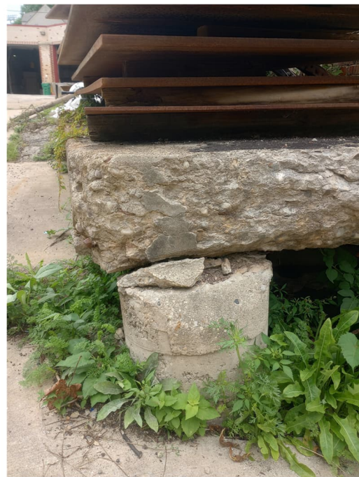
Figure 31 Exterior Platform Slab Deterioration-10
