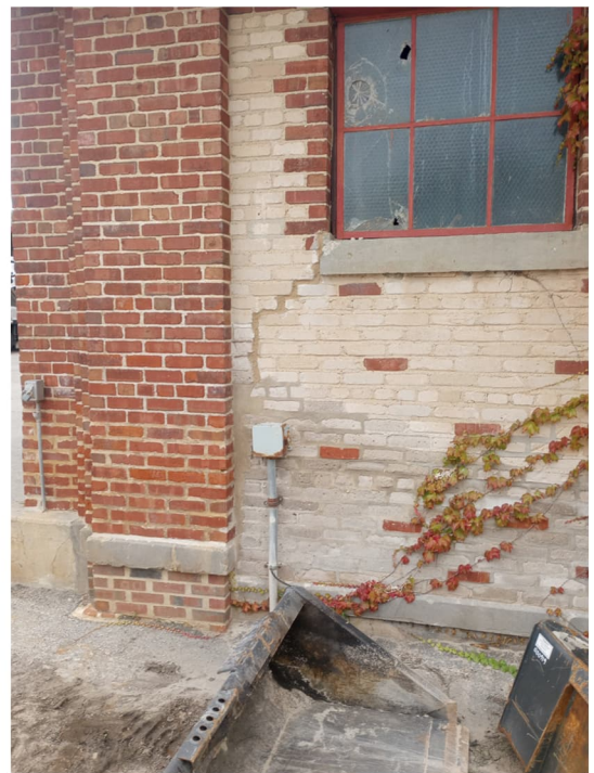
Figure 18 Previous Exterior Repairs at Northeast Building Corner
