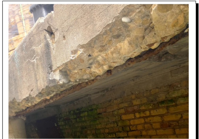
Figure 23 Exterior Platform Slab Deterioration-2
