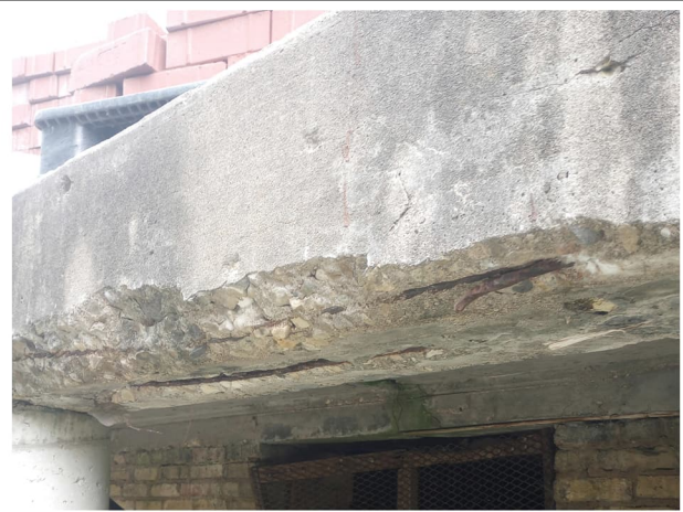
Figure 25 Exterior Platform Slab Deterioration-4
