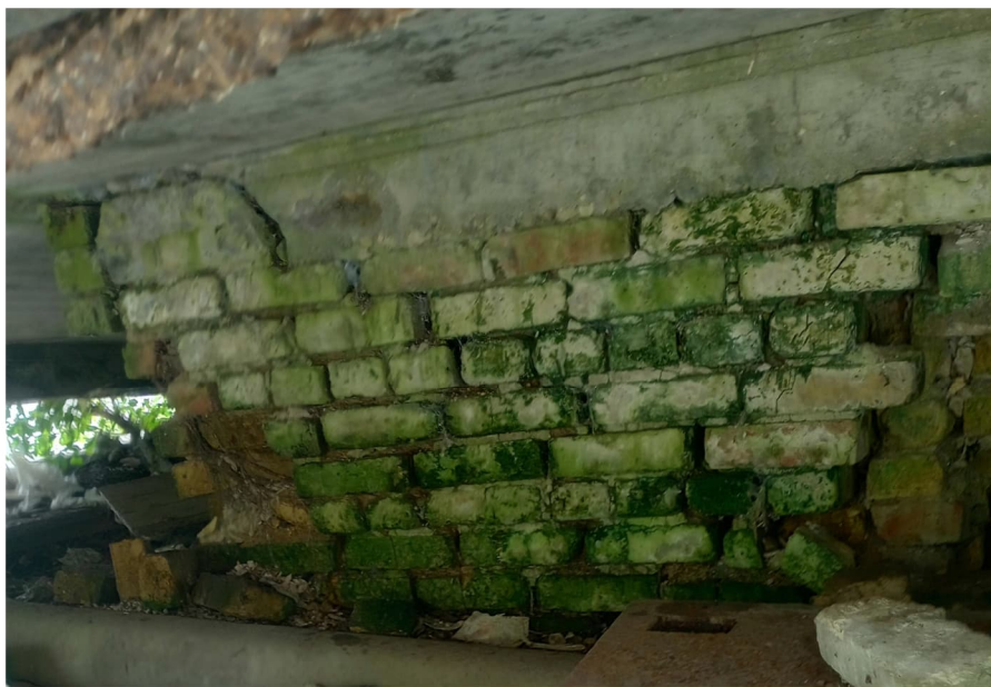
Figure 36 Collapsed Brick Foundation Wall at Northwest Corner
