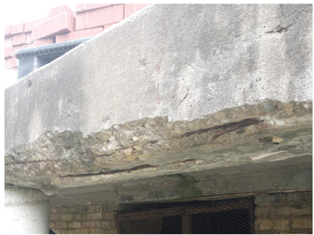
Figure 25 Exterior Platform Slab Deterioration-4
