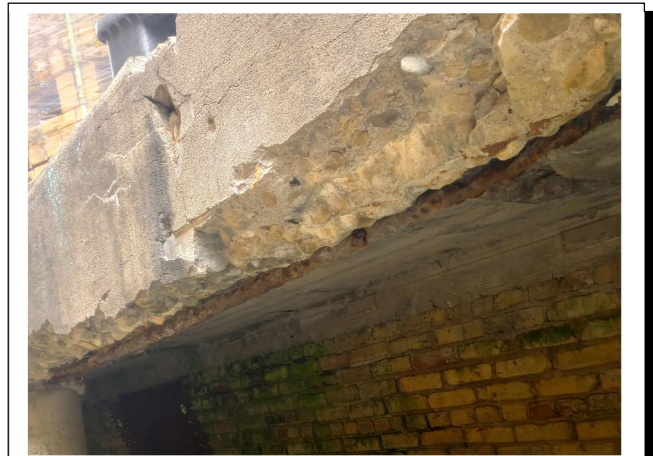
Figure 23 Exterior Platform Slab Deterioration-2
