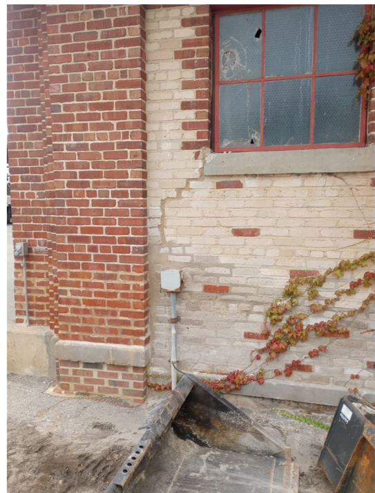
Figure 18 Previous Exterior Repairs at Northeast Building Corner
