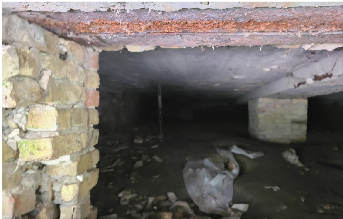
Figure 33 Corroded Steel Beam Lintel Above Access Opening
