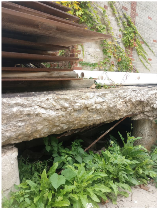
Figure 30 Exterior Platform Slab Deterioration-9
