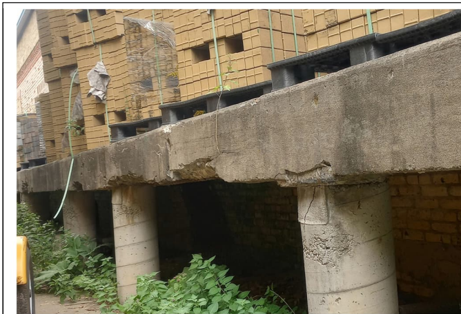
Figure 22 Exterior Platform Slab Deterioration-1
