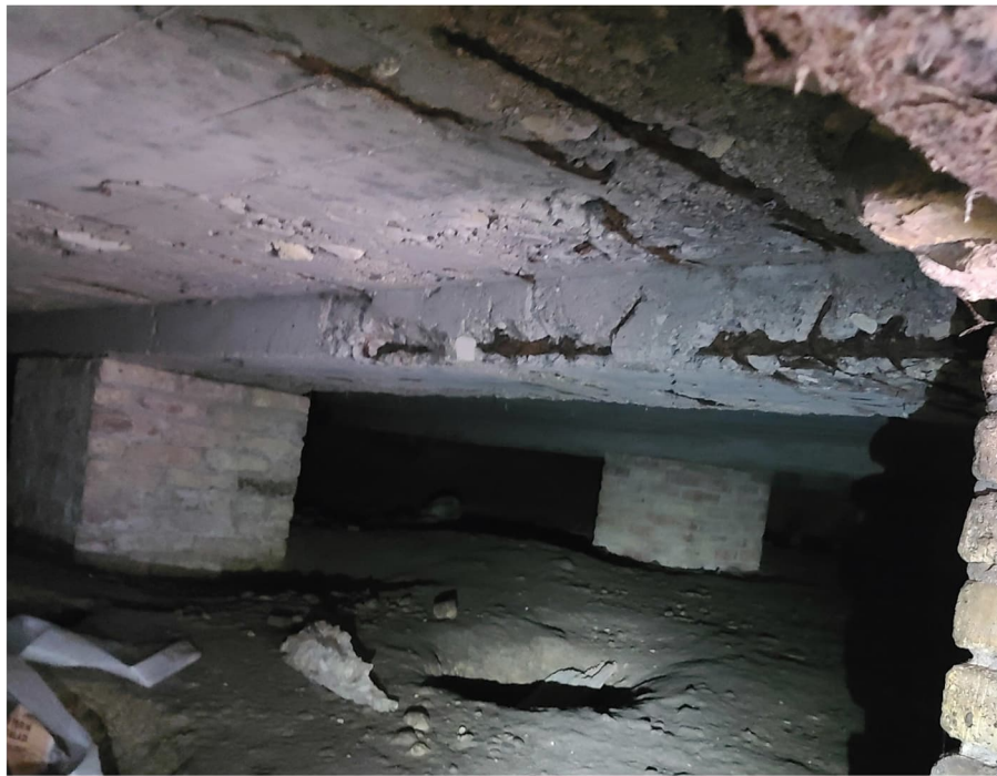
Figure 32 Concrete Delamination and Reinforcing Bar Corrosion on Underside of Building Slab
