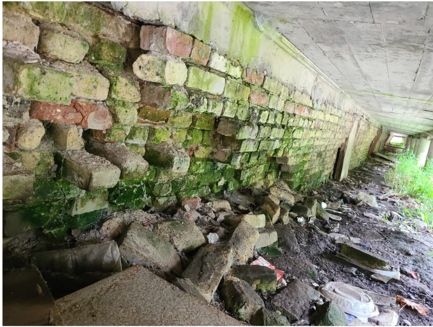
Figure 35 Collapsed Brick Foundation Wall Along West Wall
