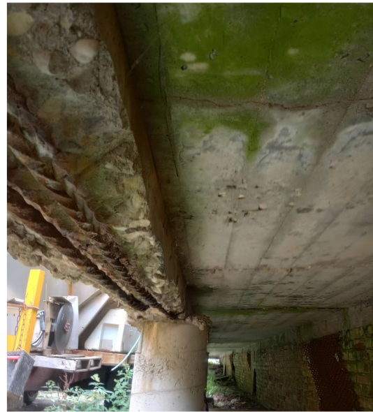
Figure 28 Exterior Platform Slab Deterioration-7
