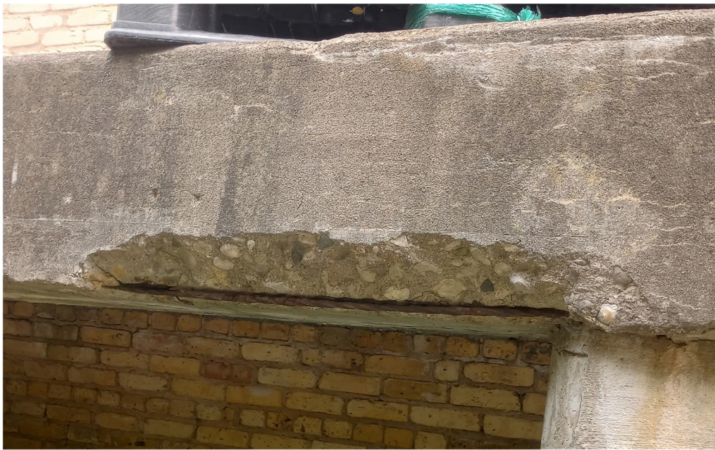
Figure 26 Exterior Platform Slab Deterioration-5
