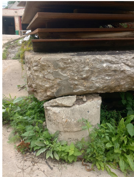
Figure 31 Exterior Platform Slab Deterioration-10
