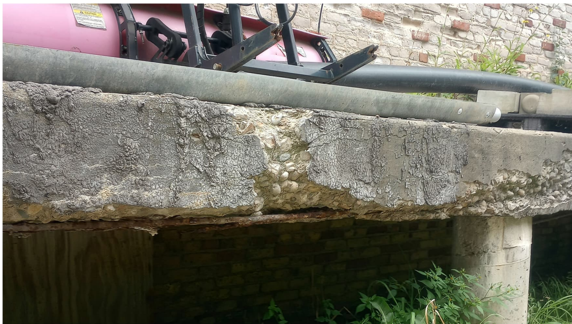
Figure 29 Exterior Platform Slab Deterioration-8
