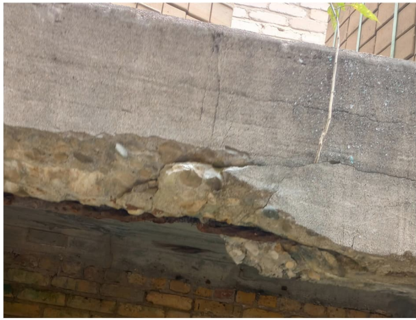
Figure 24 Exterior Platform Slab Deterioration-3
