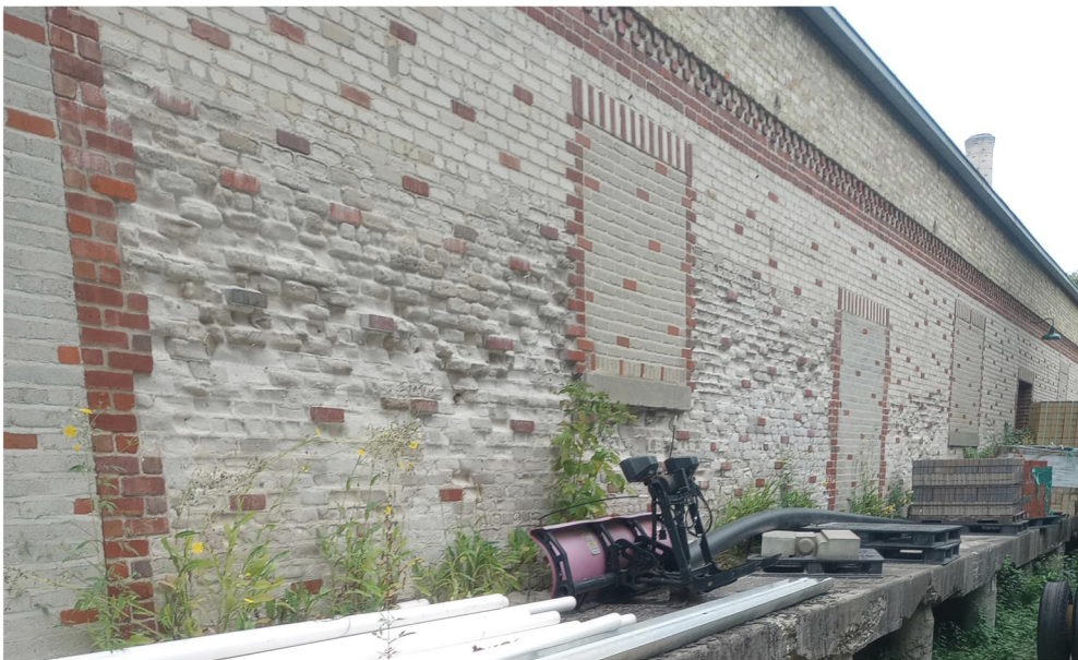
Figure 19 West Wall: Original Openings Infilled with Masonry and Significant Deterioration of Brick and Mortar Joints
