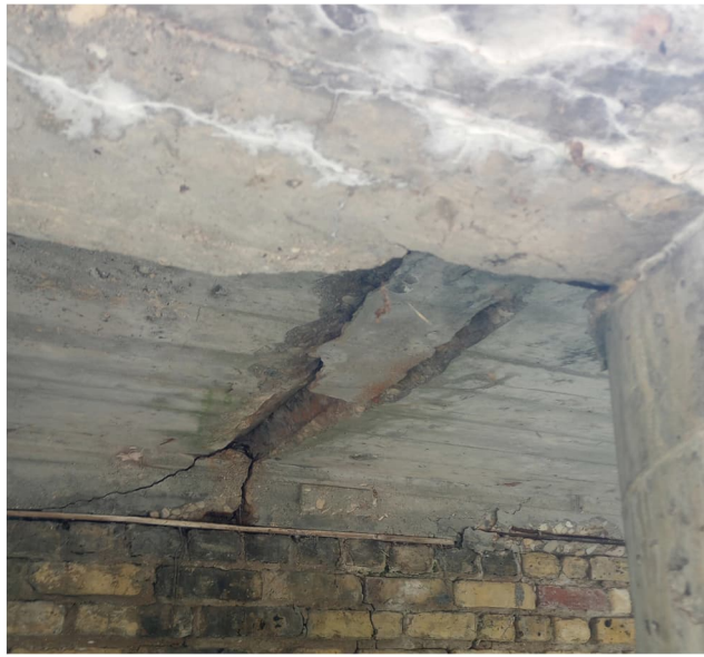
Figure 27 Exterior Platform Slab Deterioration-6
